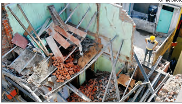
Sadar Bazar has seen many building collapses like this one last month
