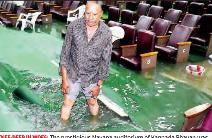
KNEE-DEEP IN WOES: The prestigious Nayana auditorium of Kannada Bhavan was inundated after Monday night's downpour. The wet spell is expected to continue
